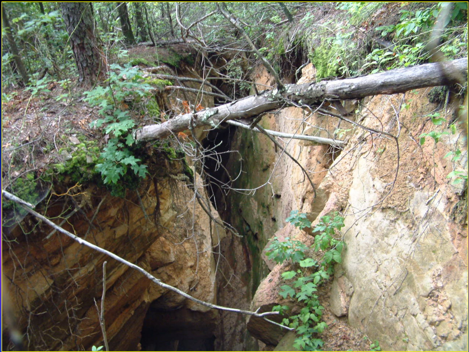
Large Land (“Mountain”) Crack
